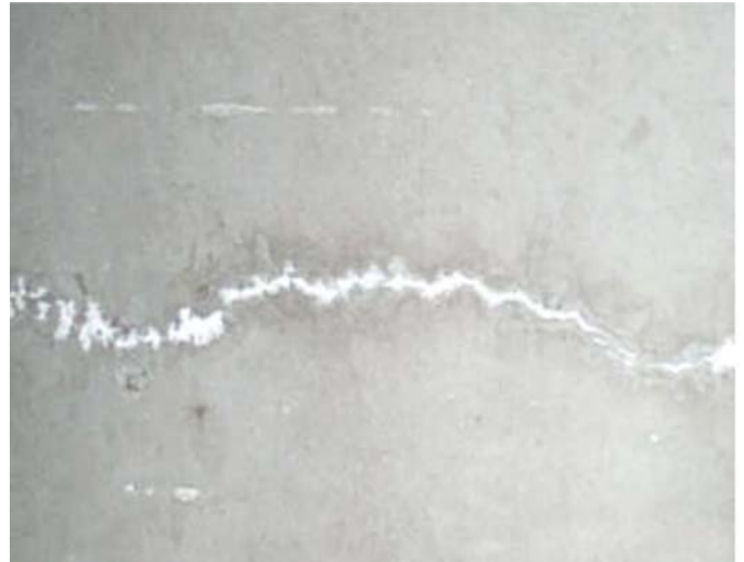
FIG. 3 Calcium Carbonate Filled Crack
